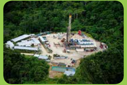
Agogo Oil and Gas Production Operator: Oil Search Ltd
