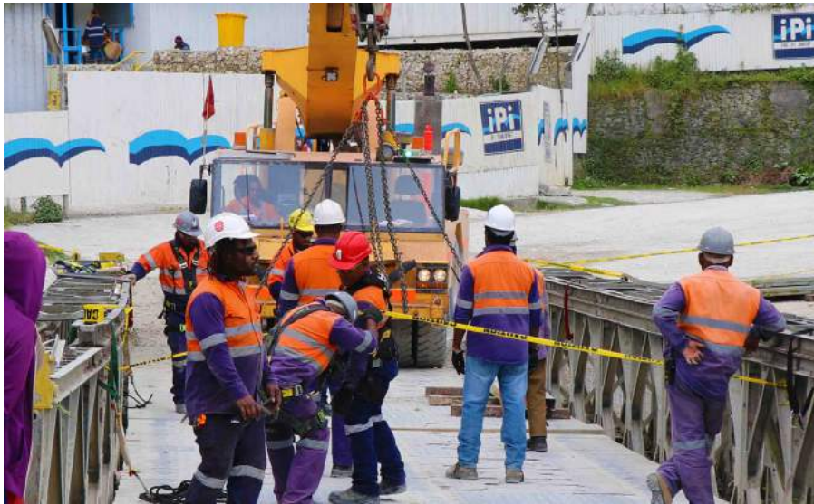
The PJV community roadworks team working on replacing deck planks at the Aipulungu bridge at Porgera Station. Pic courtesy of PJV
