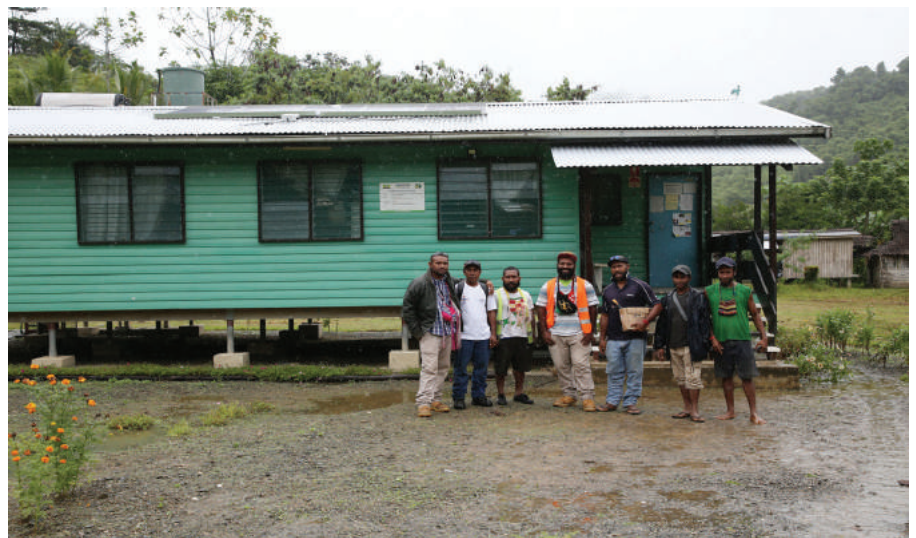
Wafi Golpu Joint Venture recently funded the renovation of the Zindaga Health Centre in the Morobe Province. The project which was completed in June this year saw the installation of an electric water pump, five solar panels, six batteries and a 5KVA inverter that can power the whole aid post. Pic courtesy of WGJV
